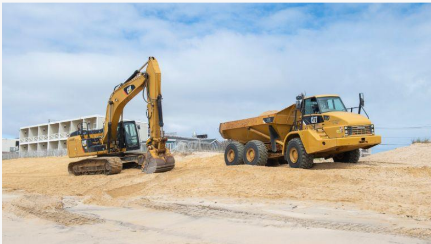
Workers used heavy machinery in May to complete an East Hampton Town sand replenishment project in Montauk. Photo Credit: Gordon M. Grant
