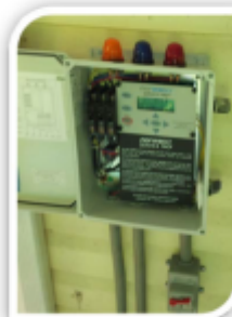
Standard I/A OWTS Control Panel
